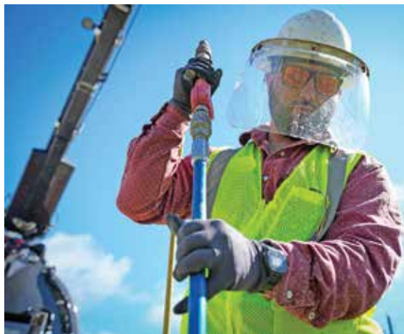
Sporting a hard hat and safety shield, Feerick uses the digging wand to pothole for utilities at a job site in Beaumont, Texas.
